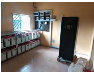
Battery bank, 60 kVA inverter, protection and control devices
